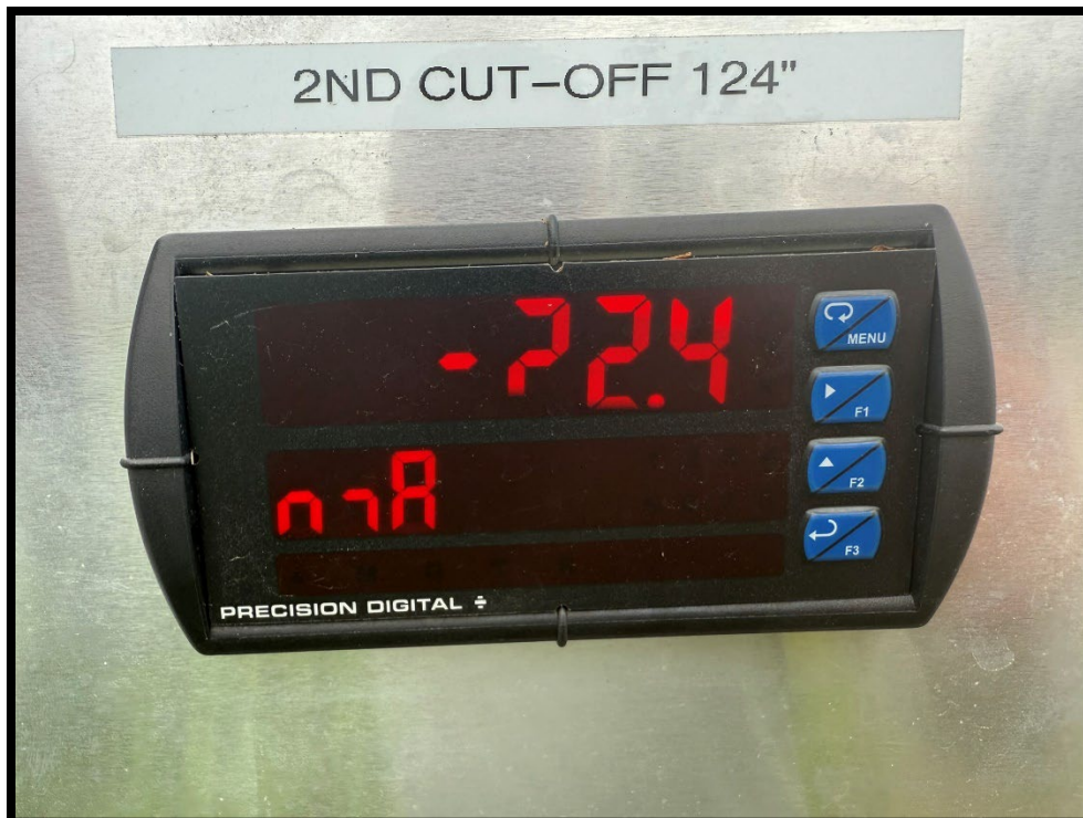
Photograph 2: View leachate tank level indicator.
